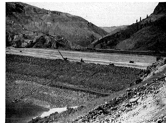
Embankment material from the borrow pits was delivered at the dam by belt conveyor, and spread and compacted by the usual construction equipment. In this photograph, the material being delivered and placed was in the impervious zone of the dam. In the foreground, the upstream slope of the embankment was being surfaced with rock for wave protection.
