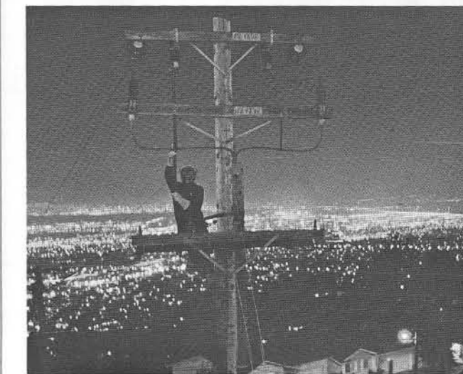
Most electric power is delivered into residential areas on 12,000-volt distribution lines like the one shown above in the hills of East Oakland, where a lineman is opening a switch. Poletop transformers lower voltages for in-home usage.
