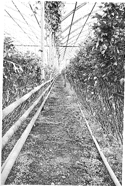
Steam Pipelines used for Radiant Heating
