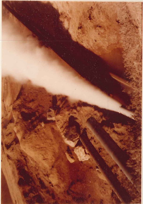
B. STEAM DISCHARGE INSIDE PIT.
