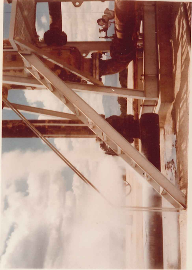
D. SEPARATOR CONTROL VALVE (CV-3) LEAK AROUND BONNET.
