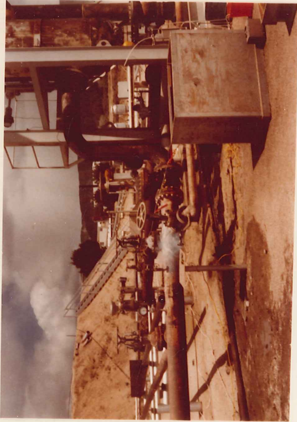
C. BYPASS VALVE (BPV-13) LEAK AROUND UNION DOWNSTREAM BPV-13.
