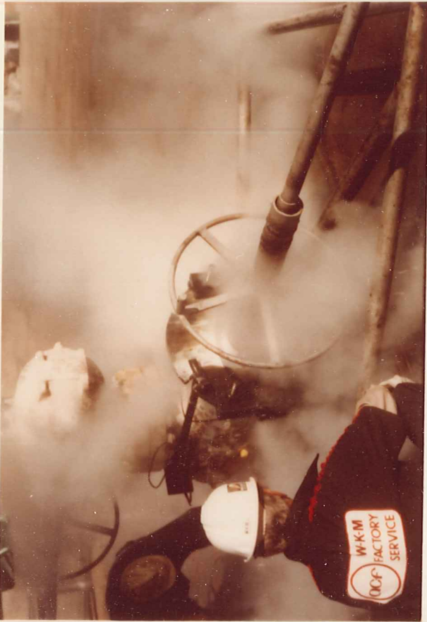
A. SAFETY BRACE NO. 1 INSTALLED ON MV-1.
