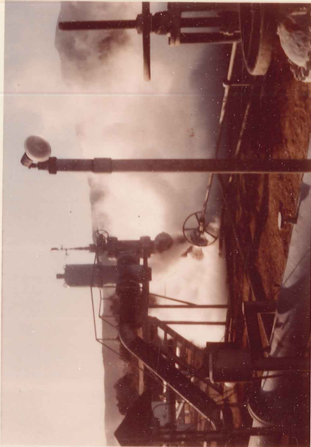
A. MASTER VALVE (MV-1) LEAKS AROUND BONNET AND STEM.
