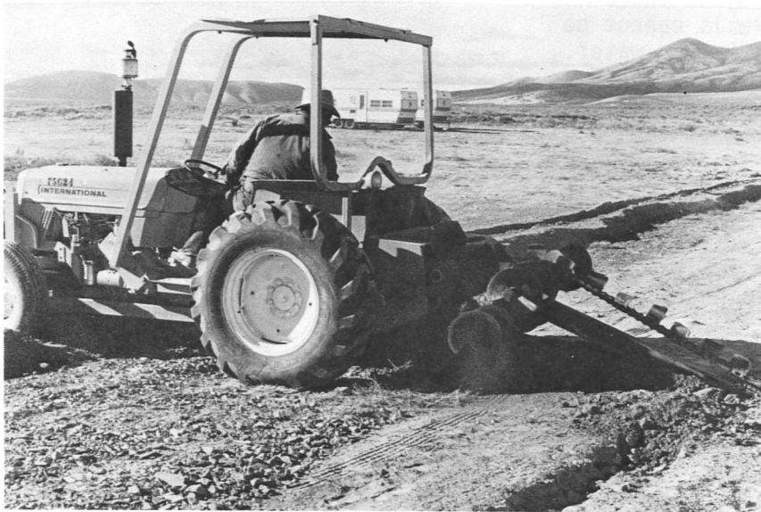
Pipelines and utilities for the various experiments and the field quarters are a major site activity. The fall weather of 1976 was particularly favorable for accomplishing the needed work. Ross Jones trenches for an electrical conduit.
