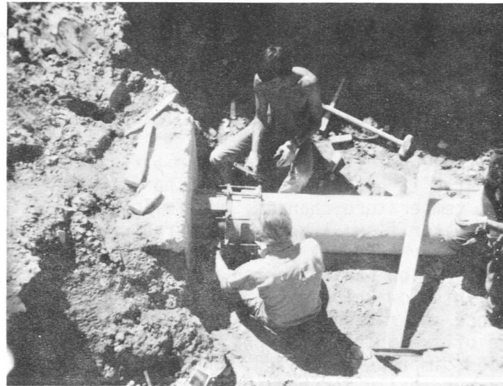
Fig. 5 Blocking Dresser coupling so that thermal cycling could not cause it to move and leak.
