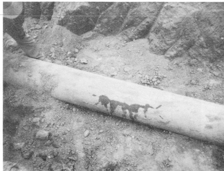
Fig. 6 Fractured line midway between sites. Reason for failure is unknown.
