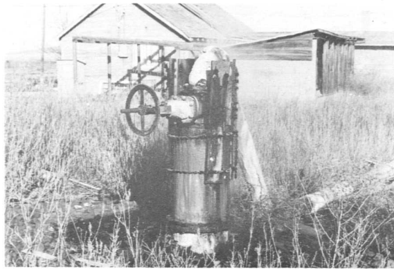
One of the 40 year old wells, now heating a greenhouse near Bridge, Idaho
